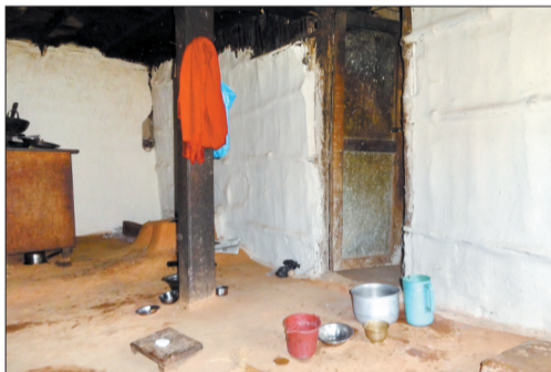
餐厅里接漏雨的瓶瓶罐罐
